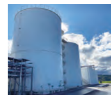
Methane fermentation equipment (Taiki Plant)
